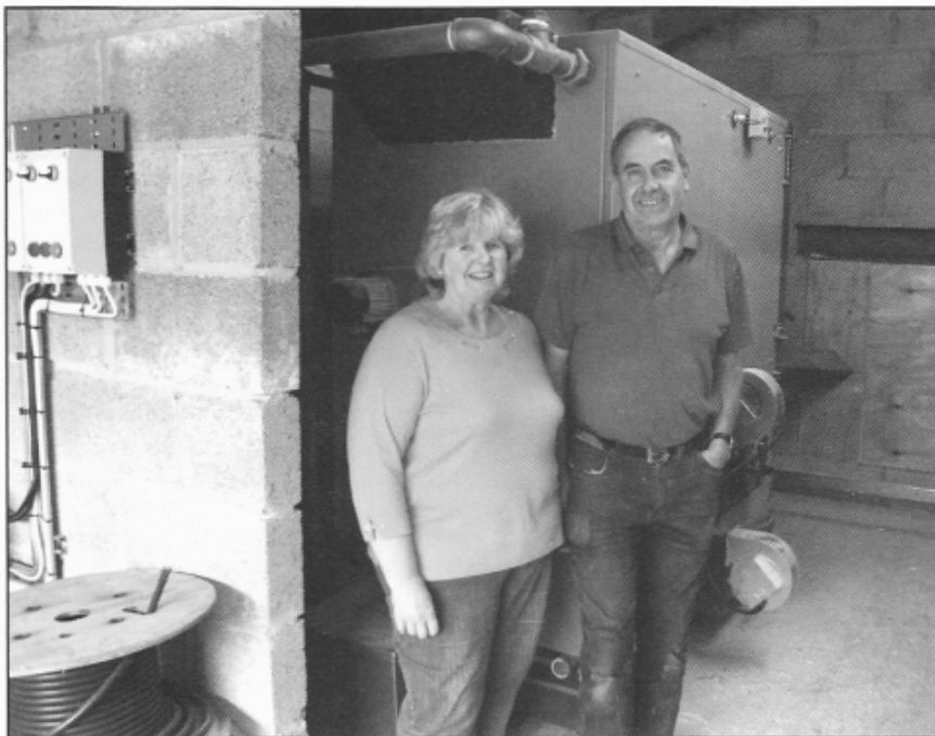
Jeff and Trish Wilson pictured by the new wood chip boiler which now provides heating and hot water for the whole Lower Gill holiday complex.
